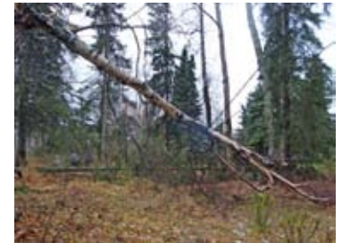
Often several trees fell across a single span of line, creating a maze of downed timber that needed to be cleared before wire could be installed.
