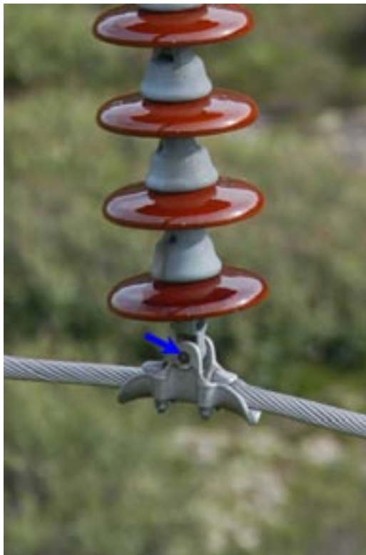
Above: The cotter pin is bent and the conductor pin has backed out to a point where it may not support the weight of the wire much longer.
