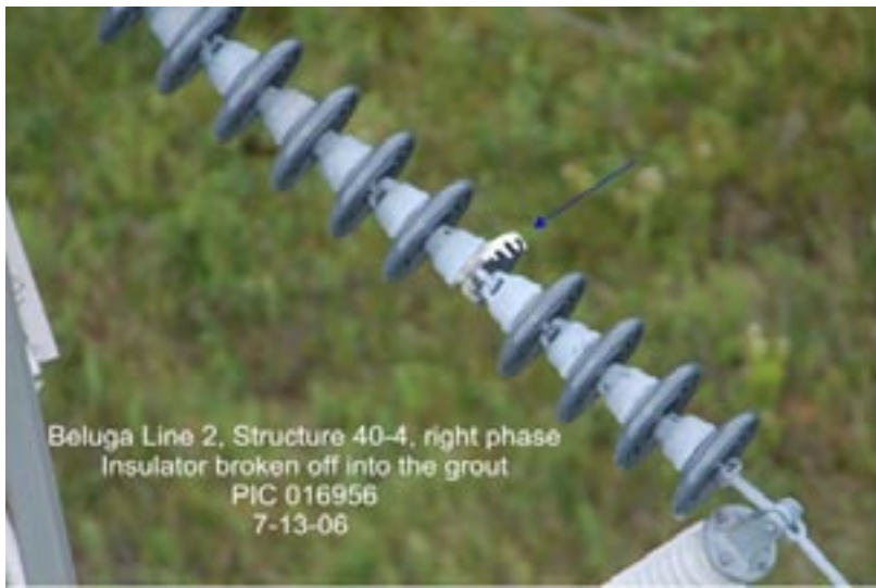
Left: This is Beluga transmission line 2, Structure 40-4, which means it is the fourth structure in the 40th mile of the line. The photo is of one of the outside insulator strings on the structure clearly showing that the fourth insulator up from the conductor has either been shot by a vandal or broken due to some type of impact or vibration.
