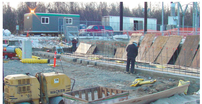
Construction is under way on the new Postmark Substation. at the north end of Ted Stevens International Airport. Chugach is building the facility to meet the increased load from commercial activity at the airport. Chugach's contractor has been excavating and constructing wooden forms for the switchgear and transformer foundations.
