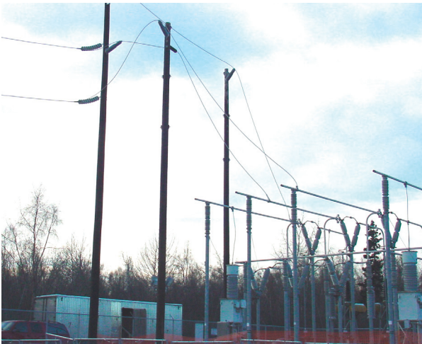
Chugach's contractor has temporarily rerouted power lines onto the structures at the left during construction of the new substation and feeder lines.
