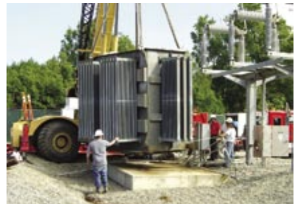
Chugach crews guided the reactor as it was moved from a concrete pad in the Pt. Woronzof Substation to a truck that brought the piece of equipment to Chugach's operations yard earlier this year.
