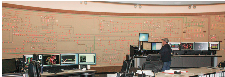
Chugach's new Outage Management System helped Dispatchers in the Power Control Center analyze and respond to outages caused by a late-September snowfall.
