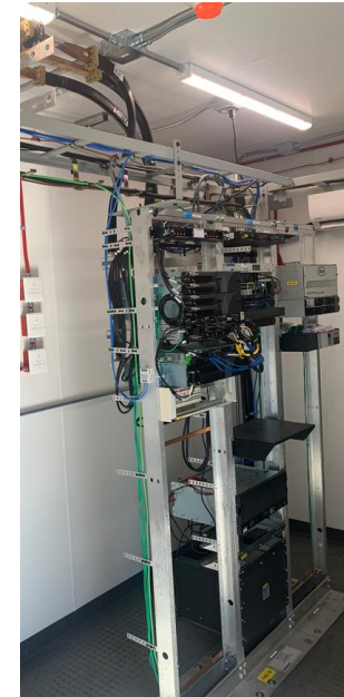
Equipment in the Enclosure
