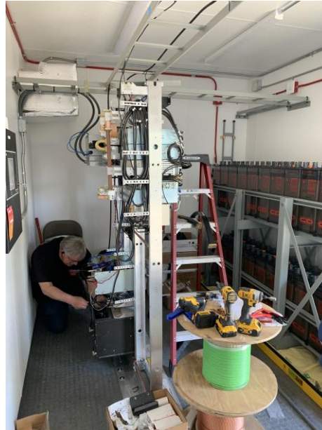
Equipment in the Enclosure
