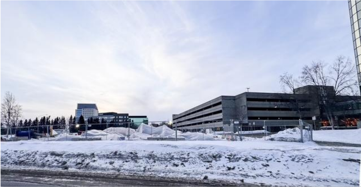
Figure 21. Construction has begun on a new hotel located on W 38 th Ave between A and C streets. The project is being developed by Peachtree Hotel Group.
