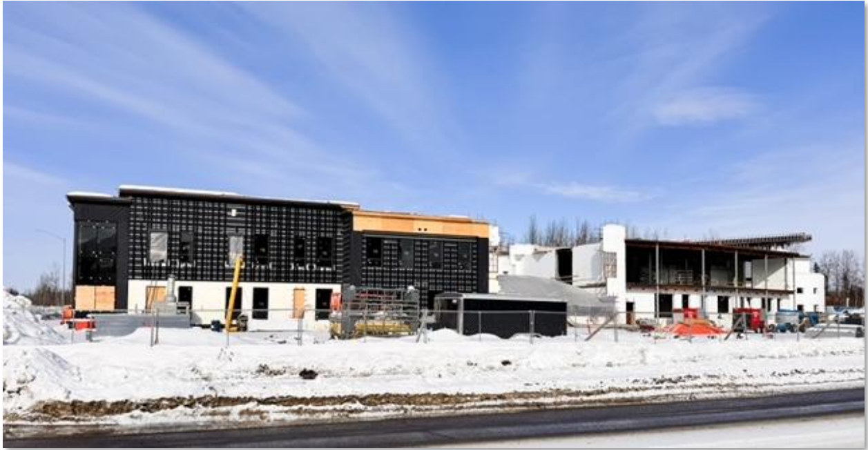
Figure 14. Construction continues for a new skilled nursing facility at the Alaska Native Medical Center (ANMC) campus. The $70M facility is over 90,000 square feet and expected to be complete in early 2027.
