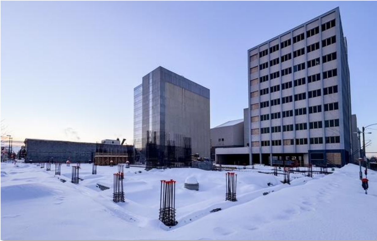
Figure 22. Construction has begun on a redevelopment project for downtown Anchorage in the block between 4th and 5th Ave. between F and G street. The estimated value of the mixed-use development is over $200 million and will replace several existing structures on the block.
