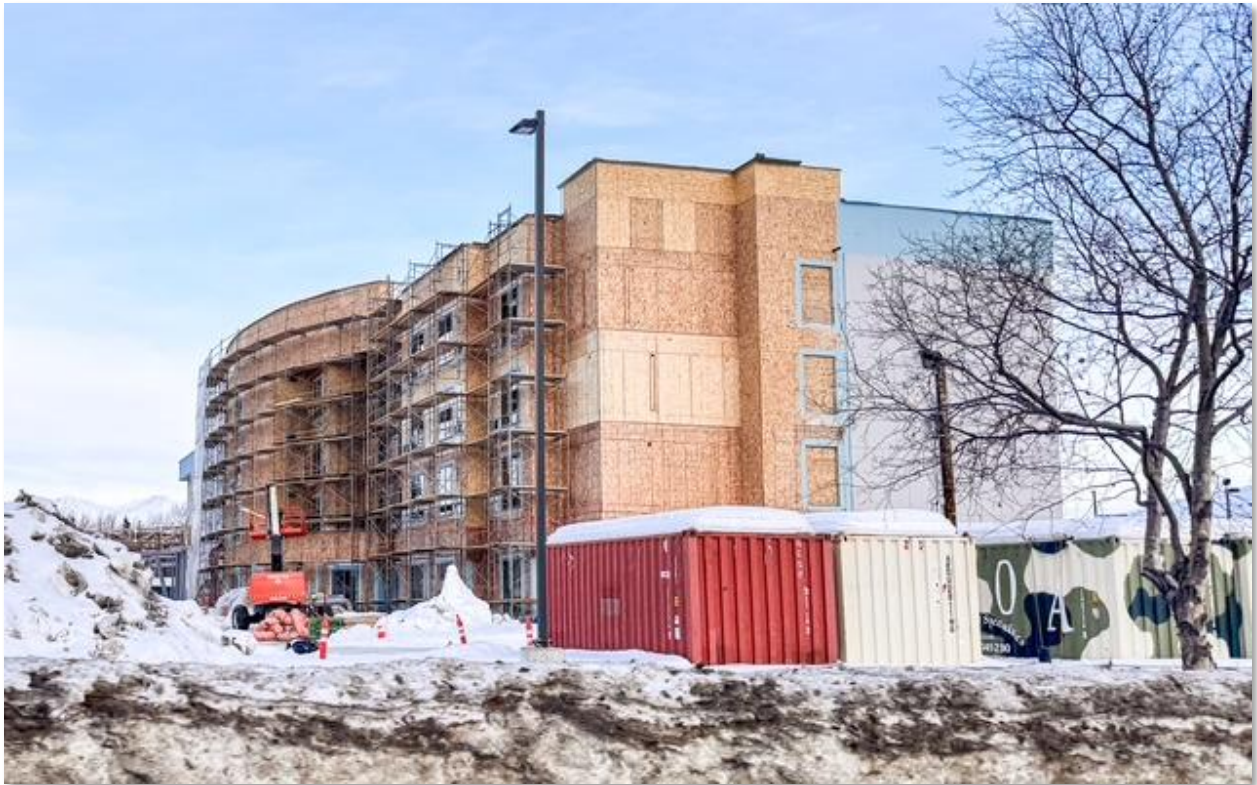
Figure 13. Construction continues for a new Courtyard Marriott in Midtown along C Street. The hotel is expected to open in spring of 2026.
