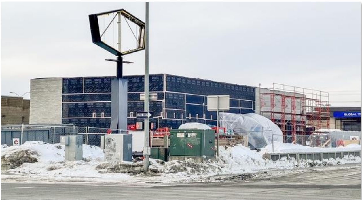
Figure 17. Construction continues a new commercial facility on the corner of Benson & Denali. The site was formerly occupied by a Denny's Restaurant that was removed in 2024.
