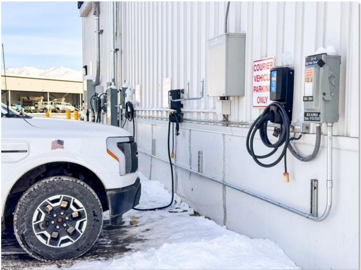
Figure 8. Level 2 Fleet EV charging site at Chugach headquarters office.
