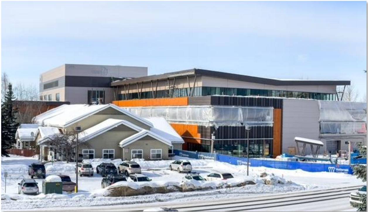
Figure 16. Construction of a new behavioral health facility continues at the ANMC campus near the corner of Tudor and Elmore Roads. The $100M facility is over 100,000 square feet and will expand the services for behavioral health and crisis support.
