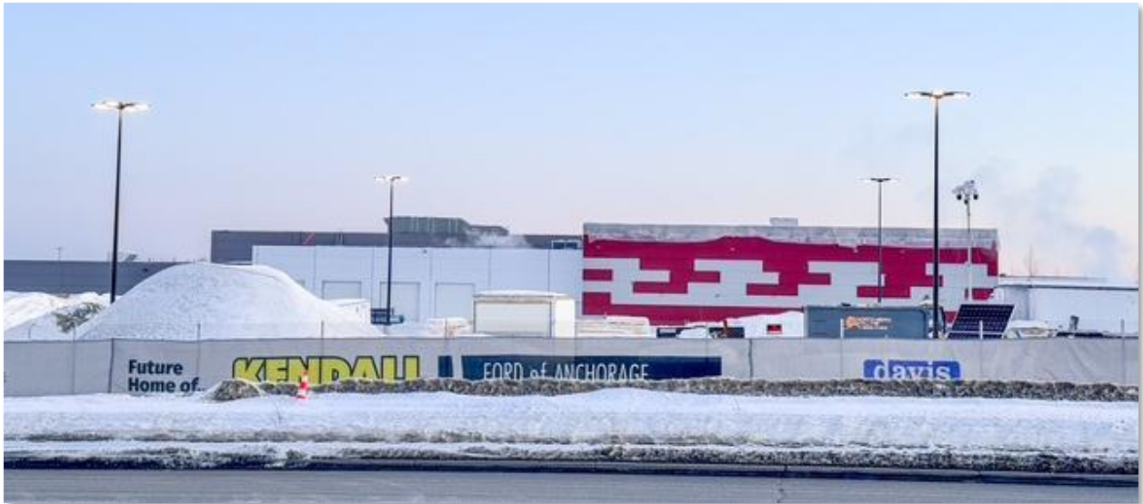
Figure 12. Construction continues for at the new Kendall Ford location near the corner of 100 th Avenue and C Street.
