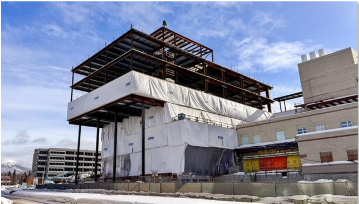
Figure 15. Construction on the emergency services facility expansion continues at the ANMC campus. The $257M facility will add 60 additional beds and enhance services available at ANMC. All project phases are expected to be completed by spring of 2028.
