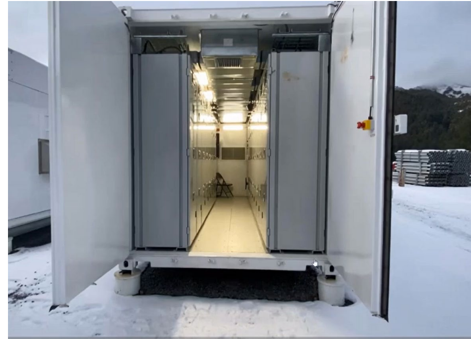
Saft developed a lithium-ion-based energy storage system rated at 1 MW with 1 MWh of energy storage capacity.
