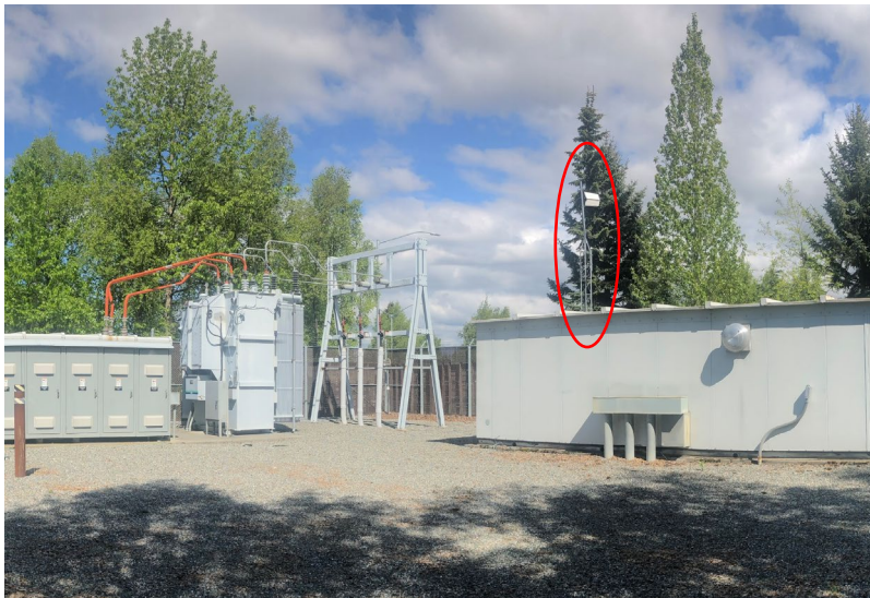
Campbell Lake Substation Communications Tower (Current)
