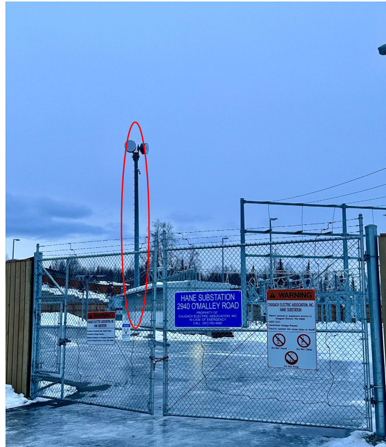
Hane Substation Communications Tower
