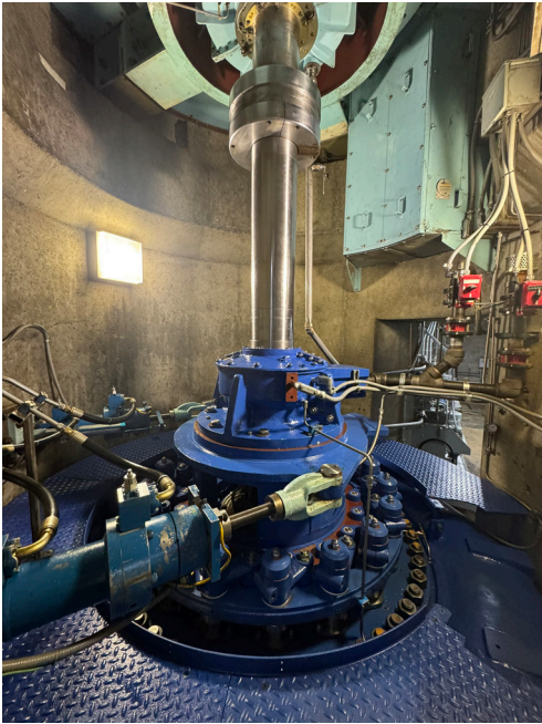
The new hydropower turbine at Cooper Lake
